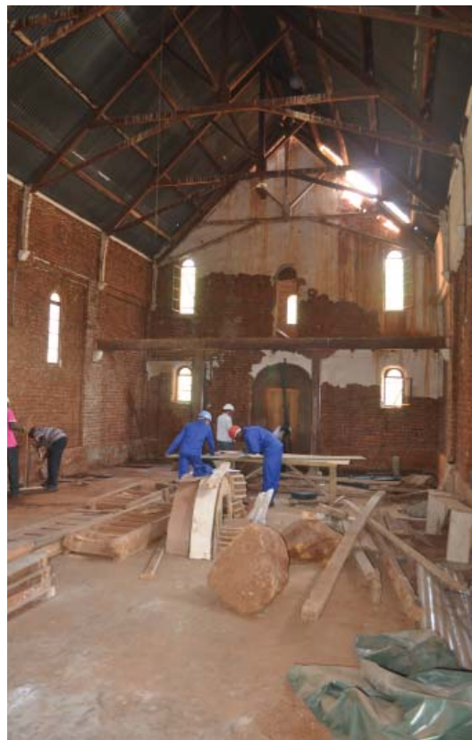
Right top and bottom: The restoration work is extensive, with parts of the building having to be reinforced, and in the case of the high steeple tower, virtually rebuilt. Restoration work is expected to be completed by July 2012.
